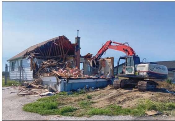
The former main terminal building at the Gore Bay-Manitoulin Airport was demolished last week. The air terminal building was first constructed in 1947. The demolition of the building was carried out as part of the major upgrade at the airport, including the opening of a new terminal building.
