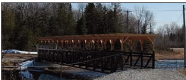
The new High Falls Bridge in Assinack township is still closed to the public due to safety precautions. However, the bridge is expected to be open by the May long weekend.
