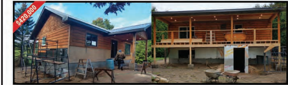
New under construction, will be finished, walkout downstairs. Double garage and storage. MLS® X5919892
