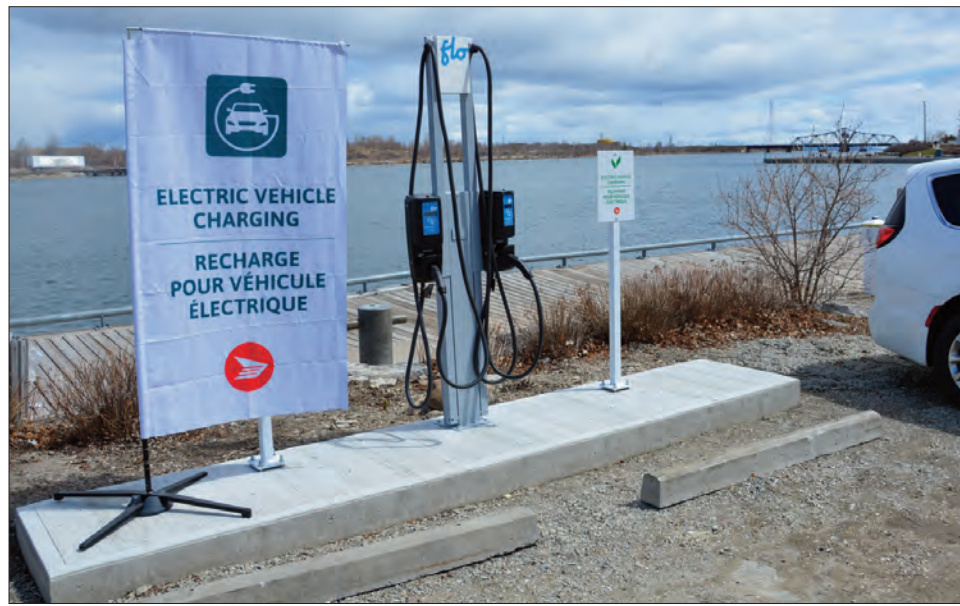
An electric vehicle charging station located in the post office parking lot is another addition to the new post office model.
