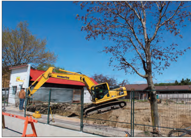
Work began on the current vacant space on the former Robinson Supply Building property on Meredith Street in Gore Bay, last week. Manitoulin Transport purchased the former building in 2019 and tore it down. Construction on the new building which will include commercial space and apartments will begin in earnest this week and is expected to be completed by June, 2024.
