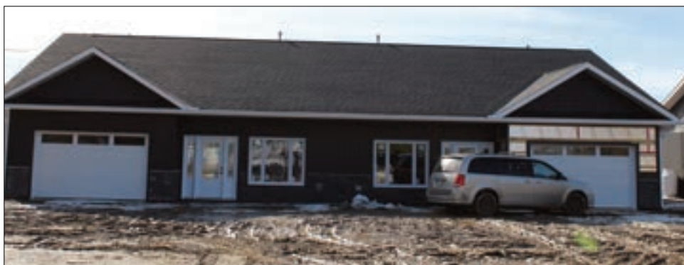
One of the three new duplexes currently under construction in the town of Gore Bay. The development is nearing completion with a mid-May moving in date for residents being planned.
