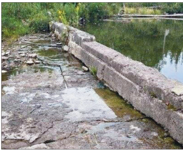
Members of the Ice Lake Landowners Association are concerned about the deteriorating condition of the Ice Lake dam, water levels and for steps to be taken to make sure the watershed is managed properly.
