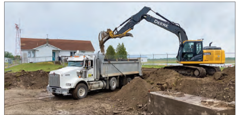
Work has now started on the major renovation project at the Gore Bay-Manitoulin Airport. Excavation work began last week and the foundation work is expected to begin this week.
