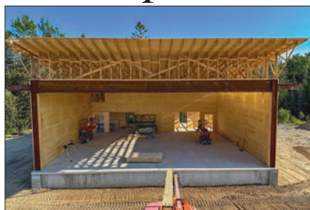
A 40' x 50' stage has just been erected at the Providence Bay Fairgrounds.
