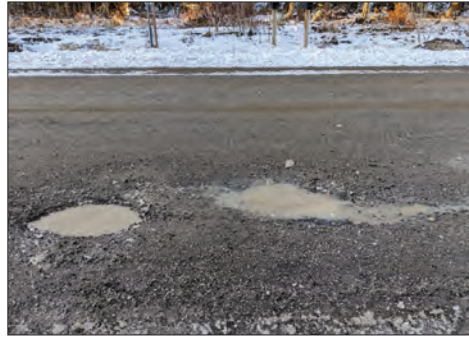
Potholes and bad road conditions like this one on the highway running through Evansville, in various locations around Manitoulin has led to concerns being raised by several residents on Manitoulin Island this spring.
