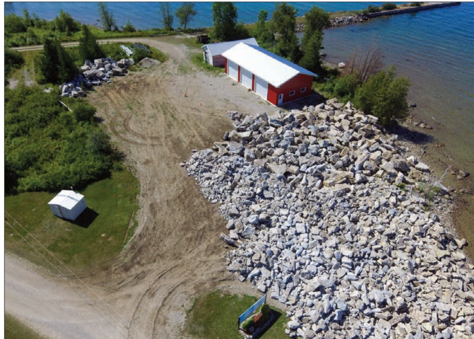
A growing rock pile at the Cockburn Island waterfront stands ready for use in a new marina break wall project next year. Cockburn Island had originally received funding for a project to fix and improve the safety of a potentially dangerous road in the community which will be completed this fall. As part of a second project, the township is using wasted rock from the road project to protect its marina from the North Channel winter ice, with the break wall project. The latter will take place next summer.
