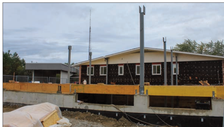
Work is continuing on the Mindemoya Hospital emergency department renovation expansion project.
