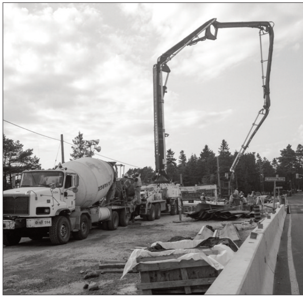
Massive amounts of concrete are shown being pumped into the new bridge in Providence Bay, spanning the Mindemoya River close to its Lake Huron mouth. Construction has gone on all summer with one-way bypass traffic controlled by traffic lights. The concrete deck on the new structure was taking its form very quickly late last week. Bray Construction is the main contractor for the bridge rebuilding.
