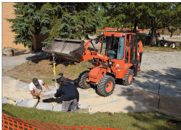
Workers carefully position a large stone slab into place in the new courtyard project at Manitoulin Centennial Manor.
