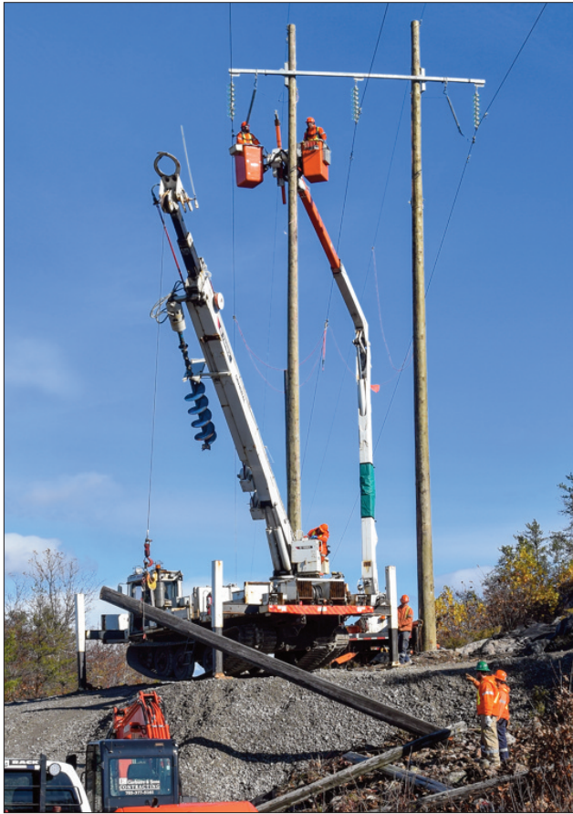
Old poles are unpredictable, so down they come. The new poles have been patiently awaiting the transfer of power.
