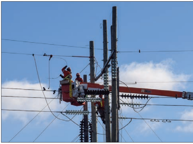
In and out of the bucket, the red seal linemen of Hydro One do what it takes to move the lines over to their new home high above Highway 6.
