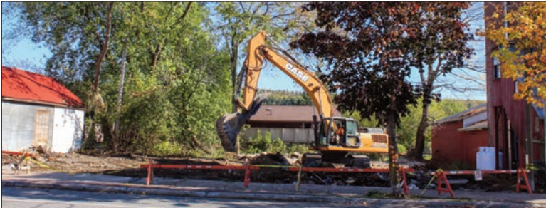
Before and after—a crew from Mike Varey and Son Excavating knocked down the Robinson Supply building in Gore Bay last week. A brand-new building with commercial space and apartments will be constructed in its place.
