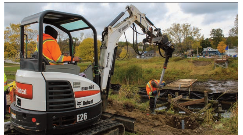
The long-awaited repairs of the Gore Bay boardwalk project have begun. The Town of Gore Bay received funding support for the project earlier this year and work permits were approved by the Ministry of Environment, Conservation and Parks.
