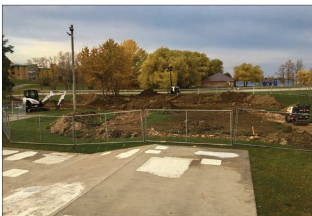
Construction on the Sisson Park pump track (BMX bike track) at Low Island is currently underway.
