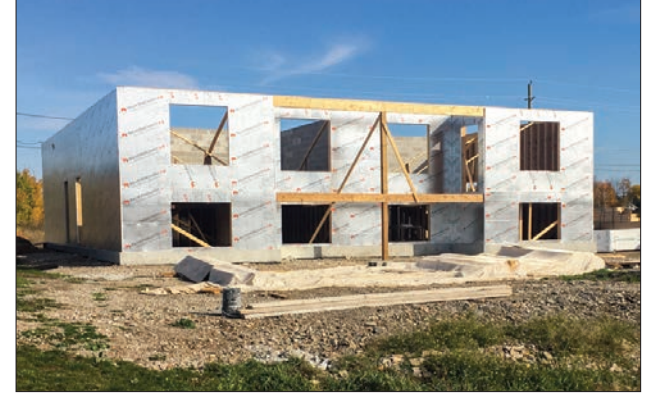
Another multi-unit building is underway in the 'new subdivision' between Hayward Street and Boosneck Road.
