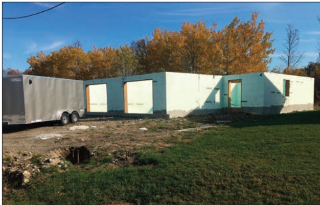
A duplex is starting to take shape in the 'new subdivision' on Hayward Street.
