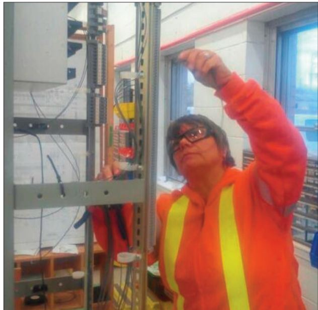
Gina Simon reviews electrical arrangement of components.
