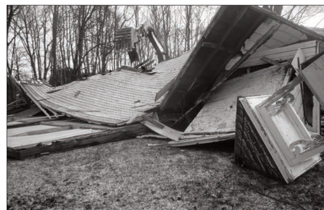
A tap of the excavator and the ancient building came down into a jumble of wood and siding
