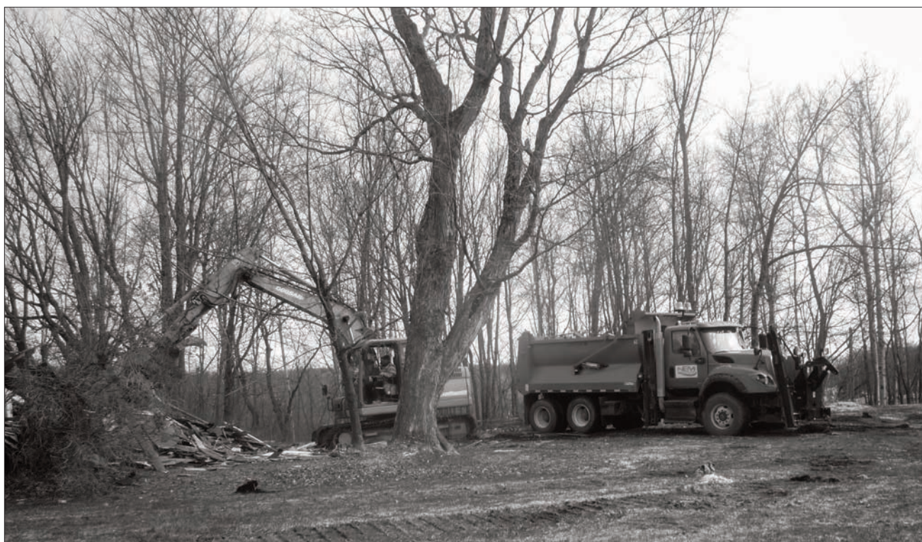
In a matter of mere moments, the former St. Peter's Anglican Church was reduced to rubble and trucked away to make way for an expanded parking lot for the Sheguiandah Seniors' Hall.
