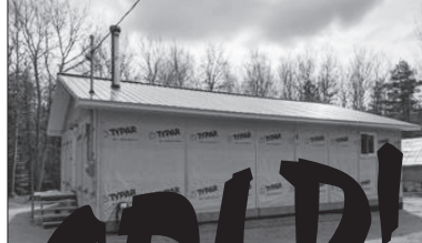
NEW COUNTRY HOME on east side of Silver Water being built on 100 ft. waterfrontage, full bath, utility room & kitchen area for kitchen dining living. Just last fall, this work in progress, is finished to the vapour barrier w/200 amp service, electric & wood heat, full crawl space, drilled well & septic. Except for some furniture, everything stays including building materials, all construction tools, 5 appliances, generator, bunkie & shed. Take a look. $129,000 (1441)
