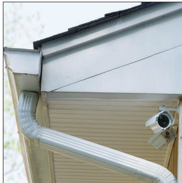
Inspect your gutters each spring. Winter storms can compromise the effectiveness of the gutters.
