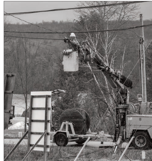
Repair crews work on fixing the downed M'Chigeeng lines on Friday afternoon.
