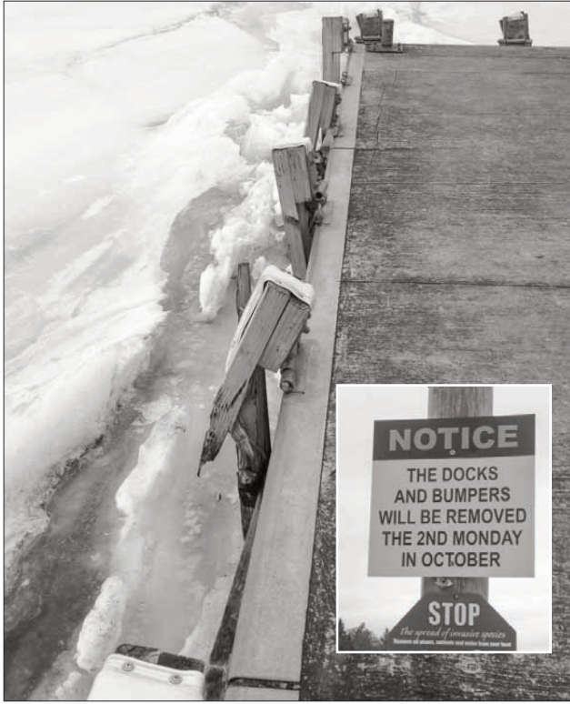
Ice damage to the bumpers lining the Sandfield public docks has one local resident seeing red.
