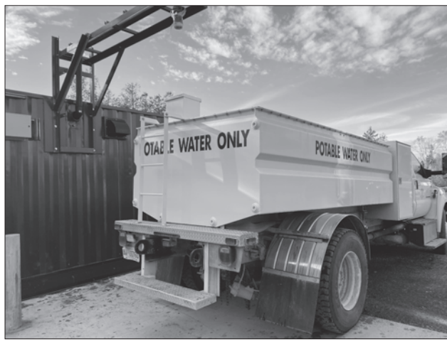
Since Zhiibaahaasing got its portable package water plant last December, a truck has re-distributed the treated water to homes.
