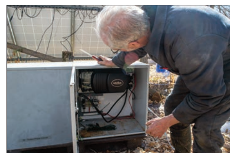
All systems are working at the solar panel array. Mr. Burt finished off the wiring process himself.
