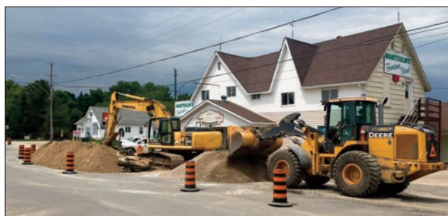
Roadwork is well underway at the intersection of Highway 551 in front of Jake's Home Centre in Mindemoya.
