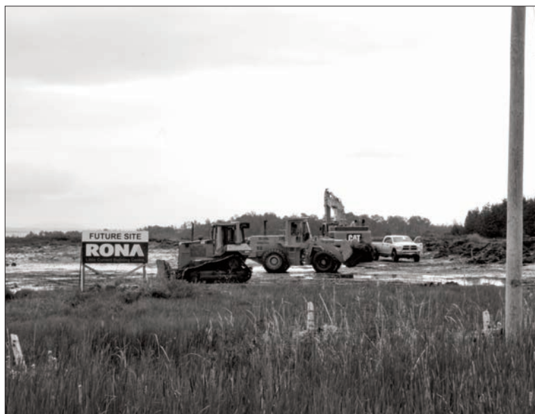
Bulldozers and a steam shovel (yes they are still called that) prepare the site for the new 20,000 square-foot RONA Little Current Building Centre facility to be built outside Little Current on Highway 6. Construction will likely be complete next March, with an opening anticipated in mid-to-late April.
