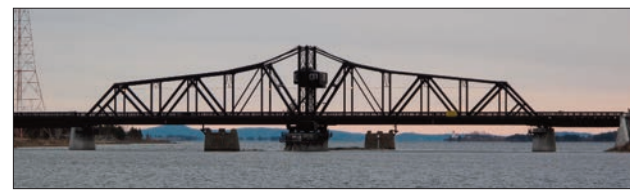
Increasingly high winds could continue to pose a problem with the bridge swings for the over century-old historic bridge.
