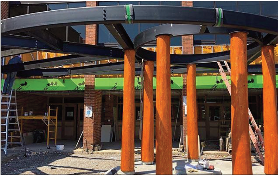
These cedar logs and upper canopy will form the surrounding area through which the steel frame will extend skyward, at the main entrance at the east side of the school.
