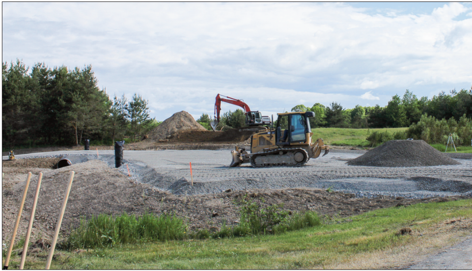
Work has started on the new parking lot to be located at the back area of the Mindemoya Hospital.
