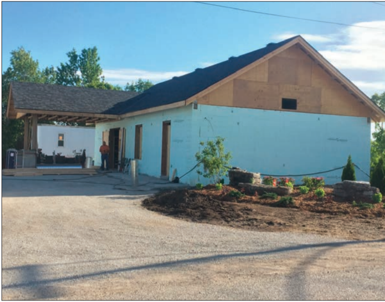
The new kingdom Hall on Wilson Street is coming along nicely thanks to the 10 to 20 volunteers that come out daily to help.
