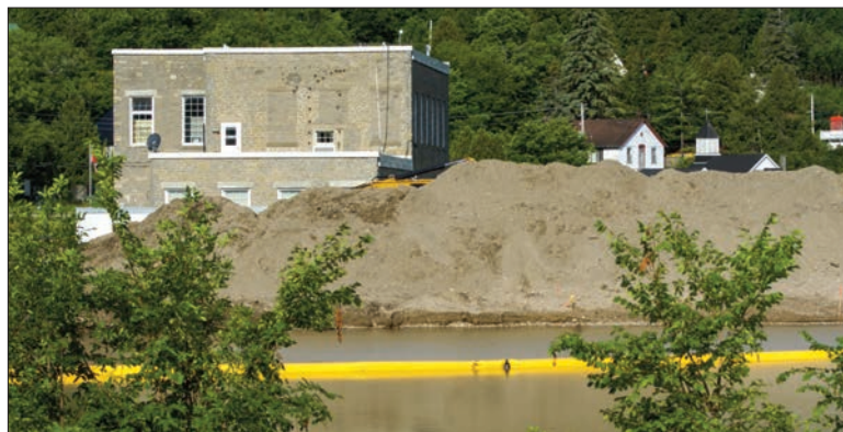
The Old Mill building hides behind sediment that has been excavated from basin. The basin will be lined with four to five inch rock and gravel will surround the perimeter of the basin for walking on. See story on Page 8.
