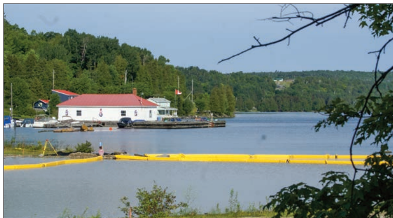
View of small craft basin construction site. Additional docks means a different 'L' shaped layout with the long arm of the L along Old Mill Road.
