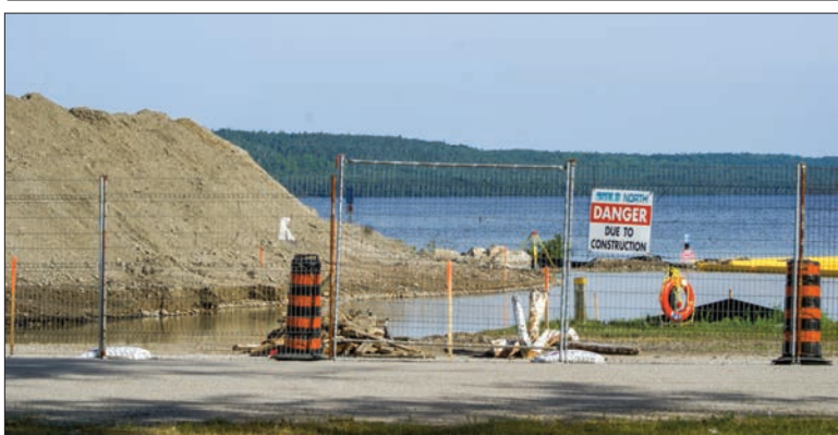
KAGAWONG SMALL CRAFT HARBOUR EXPANDING —Contractor Build North Construction Inc. has fenced off the entire small craft basin area and much of the parking lot. Lacroix Construction is also working on the project.
