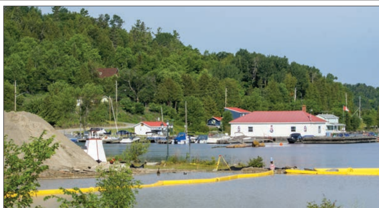
View of small craft marina construction area from Old Mill Road. The yellow barrier contains sediment from construction activities within the basin and protects the waters in Kagawong beach area and at Aus Hunt Marina (in background).
