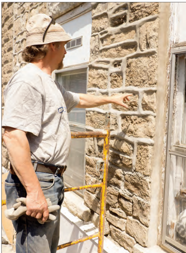
Alain Desaulniers, master stonemason, at work on restoring the mortar and limestone facade of the old Stone Block in Gore Bay, now home to two new businesses.
