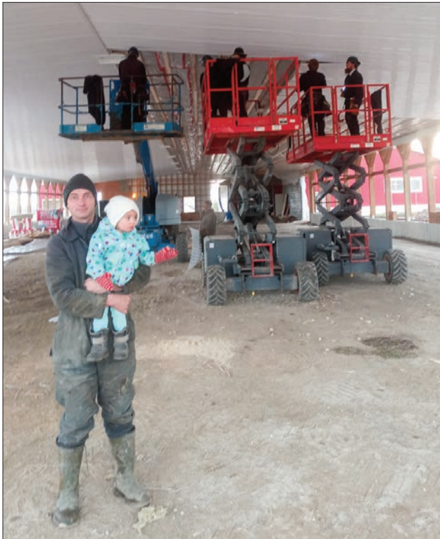
Alex Anstice and baby Chloe admire the work of the ceiling crew hard at work on December 10.
