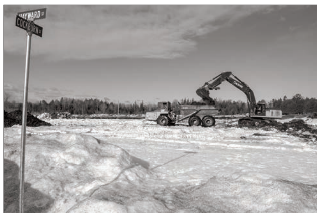
There was little to see back in April 2019 as the first shovelfuls of earth were being excavated for the new OPP station...
