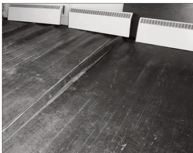
Moisture and a lack of heat in the Old School is causing hardwood floors to buckle.
