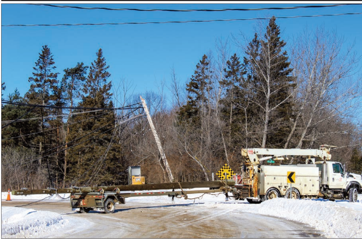
DOWNED LINE —A broken hydro pole, which brought power lines down this past Sunday morning, left a total of 5,075 Hydro One customers in the Gore Bay, Western Manitoulin, Billings, Central Manitoulin and several other areas on the Island without power for, in some cases, a lengthy period of time. The power outage took place at 7:52 am this past Sunday, with damage to the hydro pole adjacent to Wright Street in Gore Bay having broken down. While work crews with Hydro One were on scene fixing and replacing the broken hydro pole and downed lines, several members of the Gore Bay Fire Department were on hand all day and early evening, closing the road to all traffic at two locations on Wright Street and Highway 540B. Power was fully restored to all customers at 6:30 pm.
