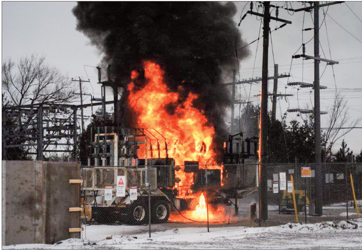
Fire rages at a Meredith Street Hydro One distribution site. The conflagration cut power to over 2,500 residents for over 15 hours on Sunday.
