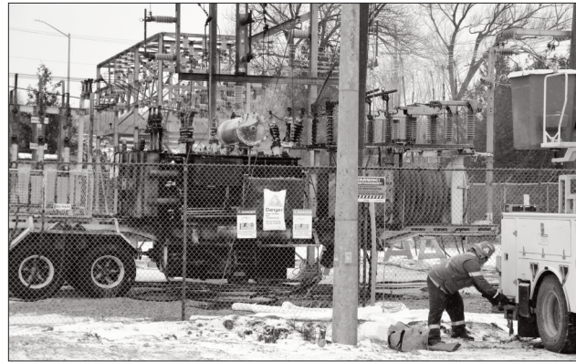
Hydro repair workers hustle to transformer station that was destroyed by fire on Sunday leaving 2,500 Island residents without power for 15 hours.
