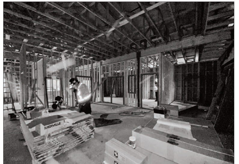
Progress inside of the expansion of the Mindemoya Emergency Department of the Manitoulin Health Centre.
