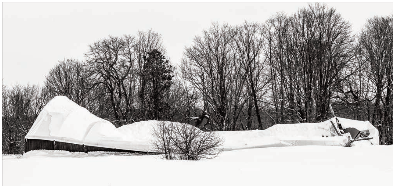
The storage structure located on the Twin Peaks Bed and Breakfast property just outside of Mindemoya collapsed from the weight of snow and ice recently, just one of many Island structures to assume such a fate.
