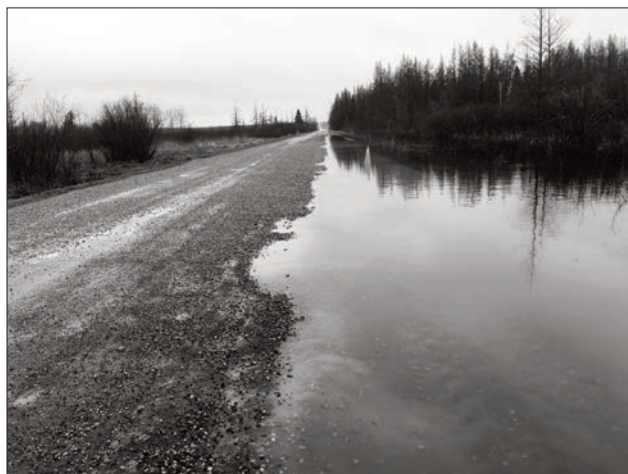
Work to the 10th Sideroad will hopefully alleviate flooding problems like this in the future.
