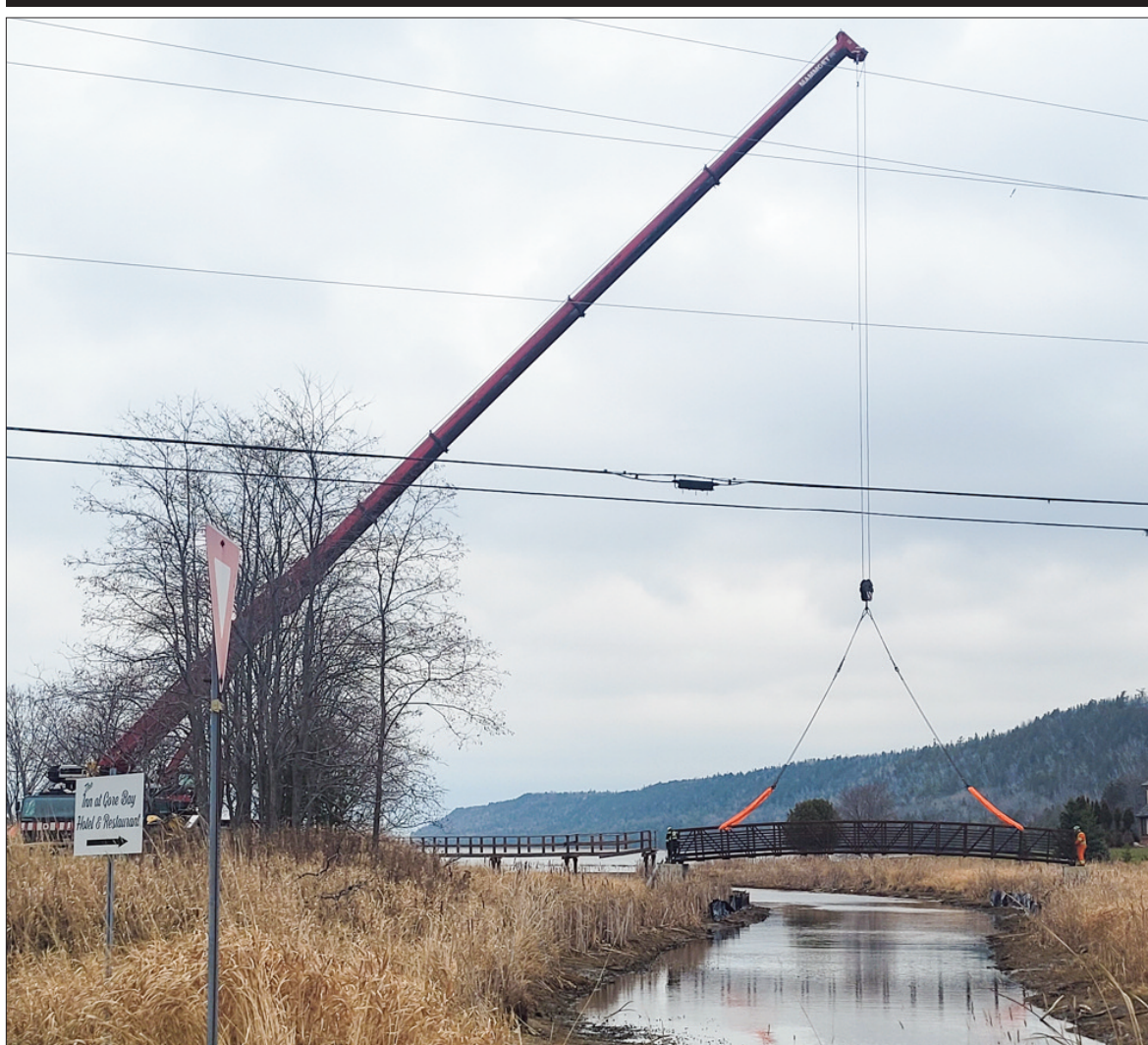
GORE BAY BOARDWALK WORK PROGRESSING —The next step into the repairs of the Gore Bay boardwalk was taken last week with the installation of two new bridges on the boardwalk. In late 2020 Gore Bay council had agreed with a helical pile (screw pile) option for the boardwalk spanning the entire portion of the boardwalk to be repaired. The repairs of the boardwalk span the west side of Water Street to the east side of Water Street.
