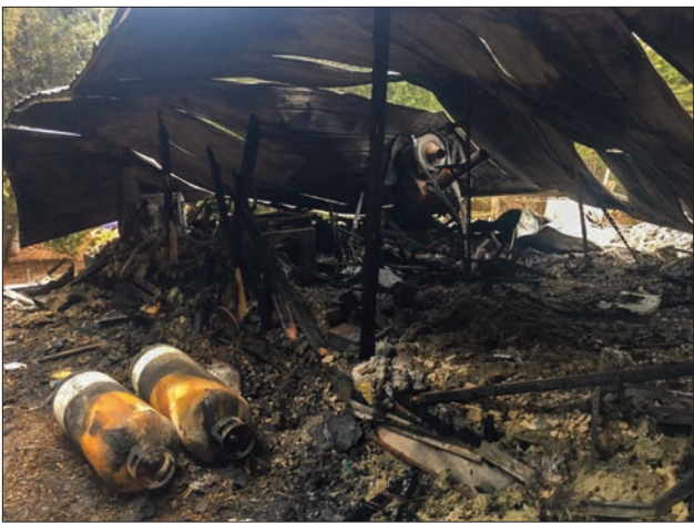
All that remains of Carol Windover’s off-the-grid Tehkummah home following a devastating November 22 fire.
