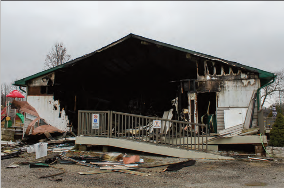
The main administration office and store, recreation and washroom facilities building at Stanley Park Campgrounds, in Spring Bay was destroyed in a fire on Tuesday, December 6.
