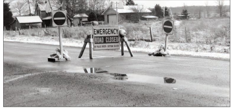
Three kilometres south of Mindemoya, Highway 542 was closed for three days due to a culvert failure last week.
