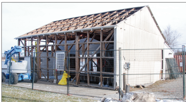
The bare bones of the OPP boathouse begin to show through as the cladding and roof are stripped off.
