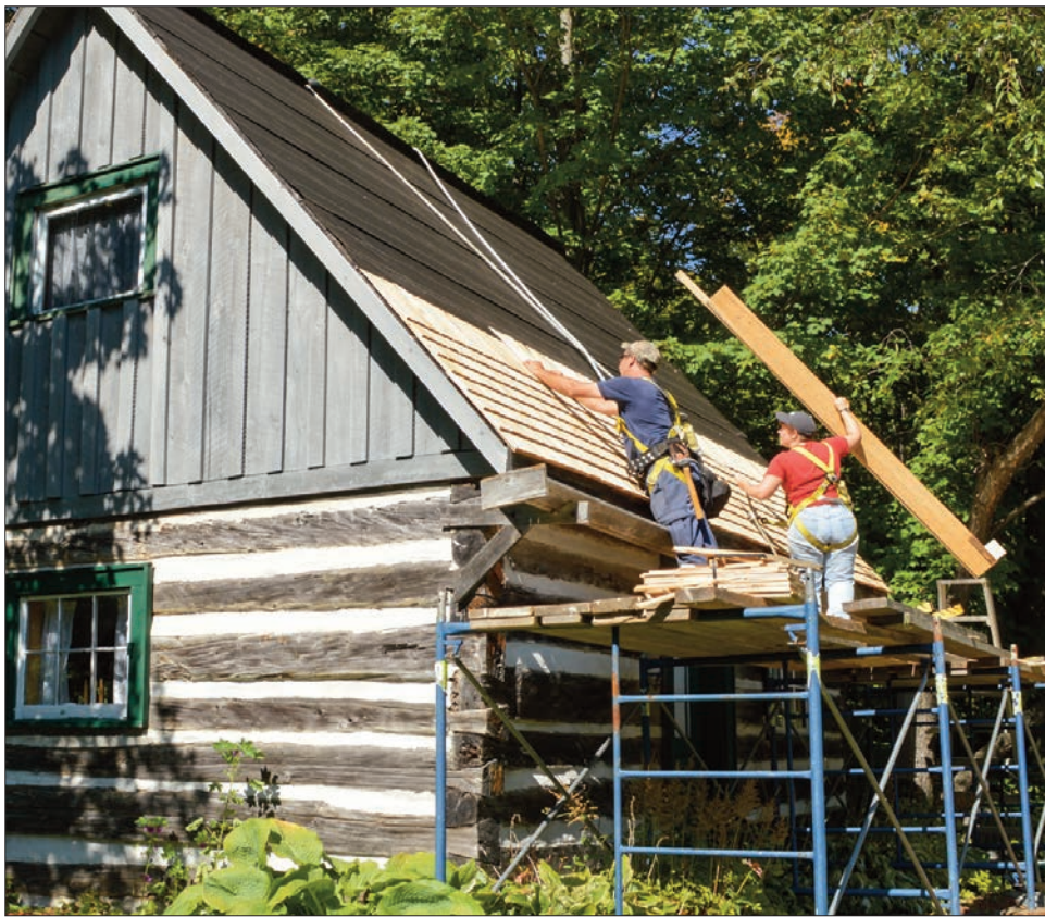
Ben and Crystal Lentir work on replacing the cedar shingles on the roof of the log cabin at the Pioneer Museum in Mindemoya.
