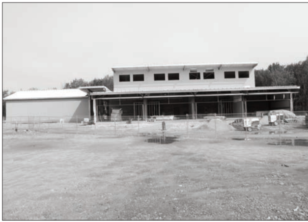
The new multi-use complex and business centre in Aundeck Omni Kaning is nearing completion with an October end date in site.
