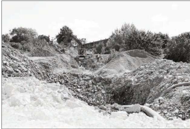
Blasting and excavation has moved ahead on the property behind Channelview Apartments in Little Current. The District Services Board is installing a new sewer line from the apartment building.
