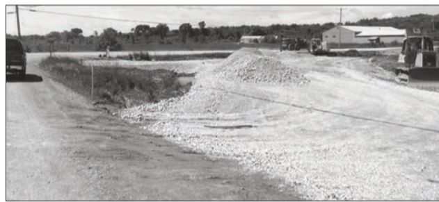
Work is underway at the new tri-intersection of Cardwell, Arthur and Meredith Streets in Manitowaning.
