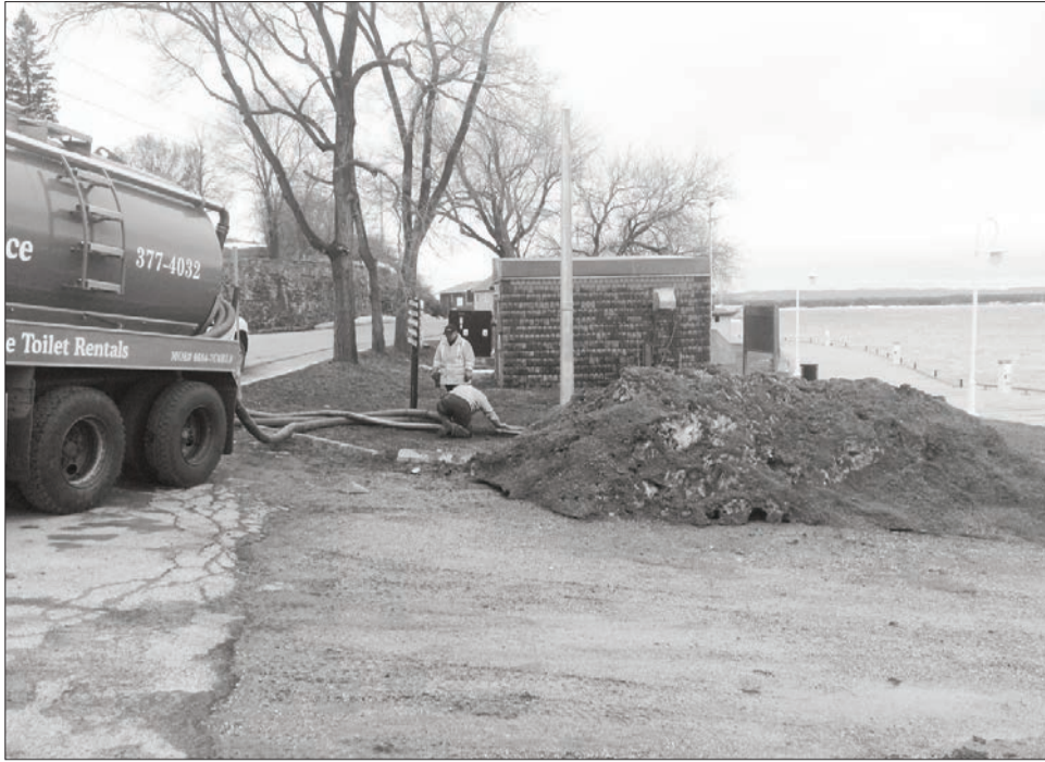
Crew works to pump out water and sewer from the storm drain last month in an effort to stop the system from overloading and backing up into the North Channel.
