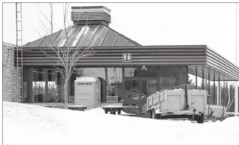
Renovations and upgrades are currently underway at the South Baymouth ferry terminal. Work is expected to be completed in April, before the start of the 2014 Chi-Cheemaun season.
