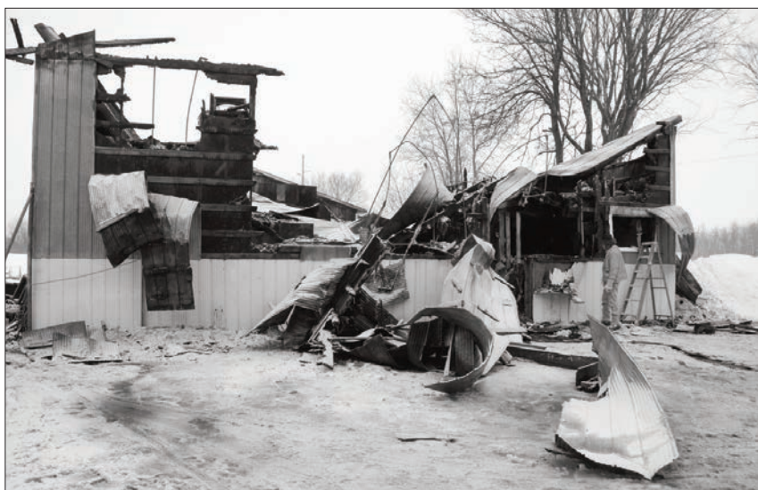
Northeast Town public works employee Dave Draper peers into the wreckage where the manager's office once stood.
