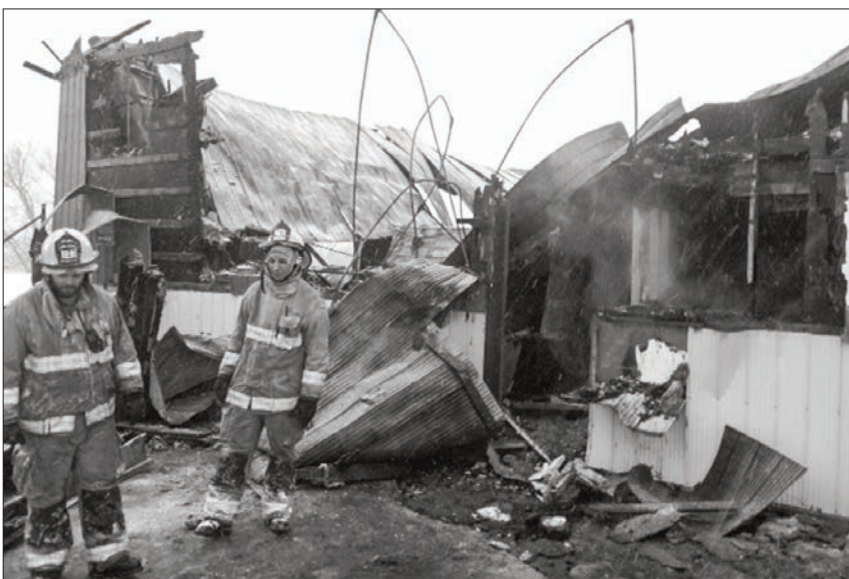
Firefighters with the Northeast Town fire department worked throughout the night and morning last Thursday to stop the blaze.
