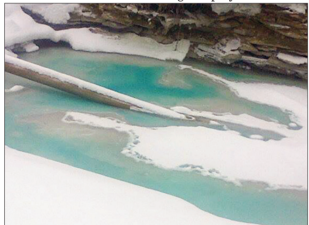
This boring hole at the McLean's Mountain wind farm project site captured on December 21 is seen surrounded by a blue/green liquid, possibly antifreeze.
