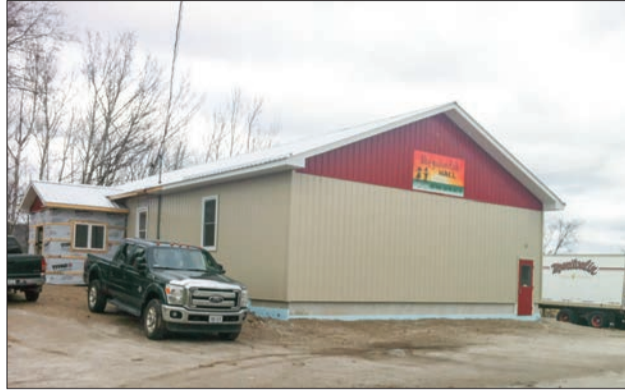
The outside of the newly renovated Sheguiandah Seniors' Hall. The work is scheduled to be completed by early December.
